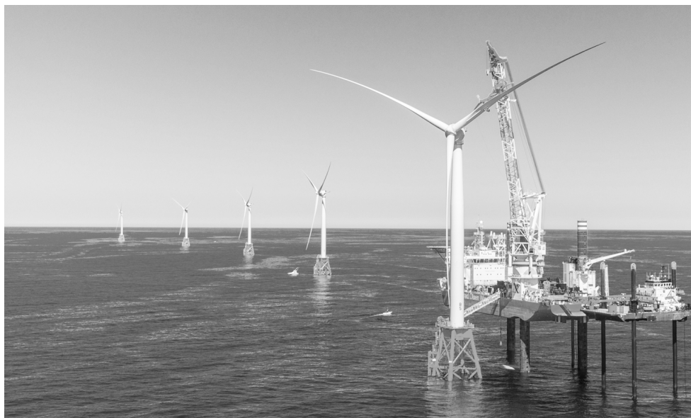
Wind turbines under construction off Block Island (photo courtesy of Deep-water Wind).
