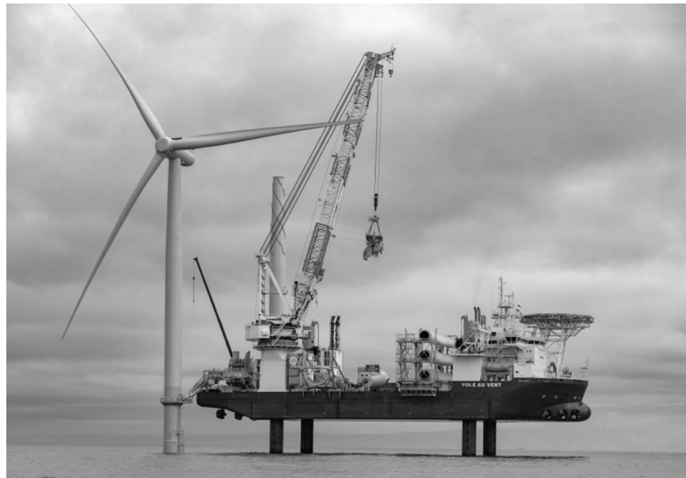
The first turbine installed in federal waters, part of the Coastal Virginia Offshore Wind project, was completed in late June 2020. The Coastal Virginia Offshore Wind project is a demonstration project developed by Dominion Energy and Ørsted (photo courtesy of Ørsted).
